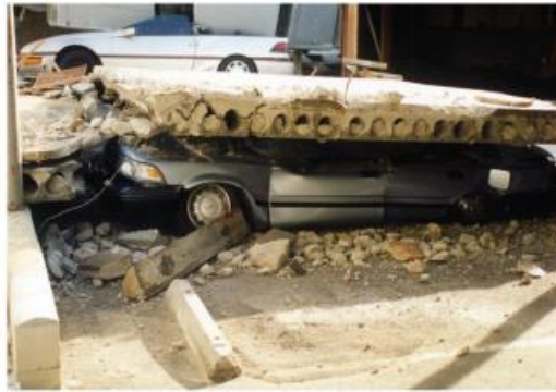
Figure 8. Hollow-core unit after the Northridge earthquake [20]
