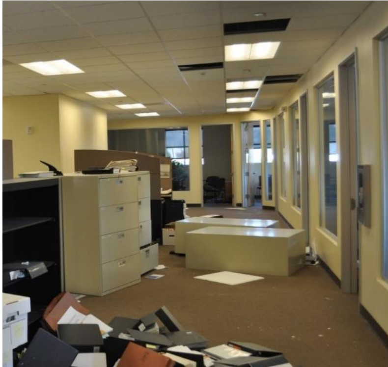
Figure 1. Damage to non-structural components in Napa after the 2014 earthquake.
