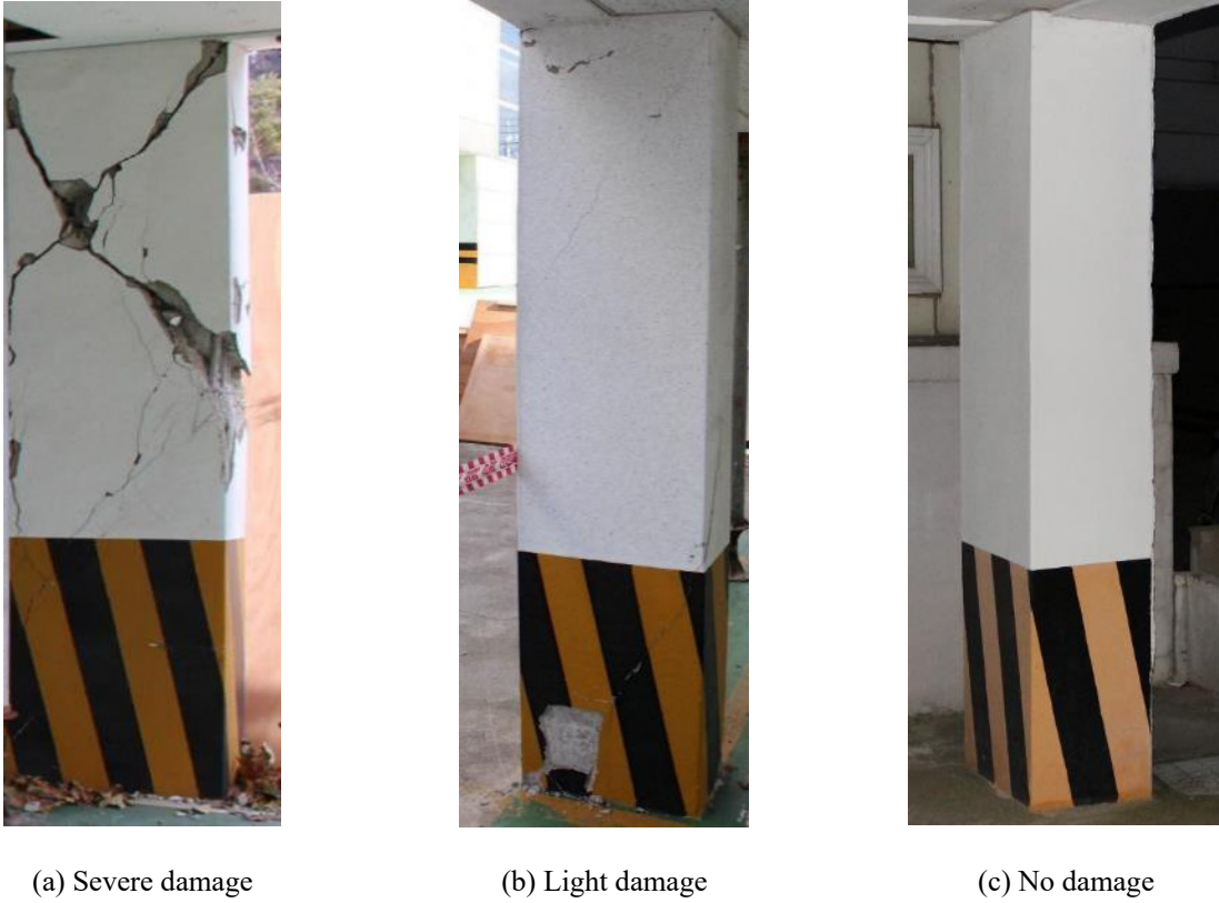
Figure 5: Images captured from multiple views of a structural column with damaged and undamaged sides.
