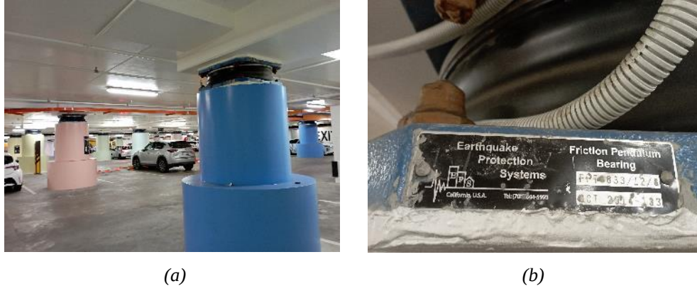
Figure 5. Photos of seismic base isolators (taken by Shen Zhan in October 2022): (a) seismic base isolators on foundations, (b) Label of a seismic base isolator.
