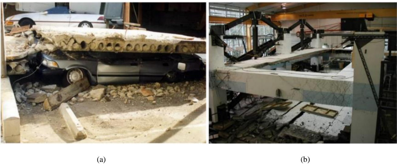
Figure 3. a) Hollow-core floor collapse during 1994 Northridge Earthquake [21] b) Hollow-core floor collapse in large-scale test [10]
