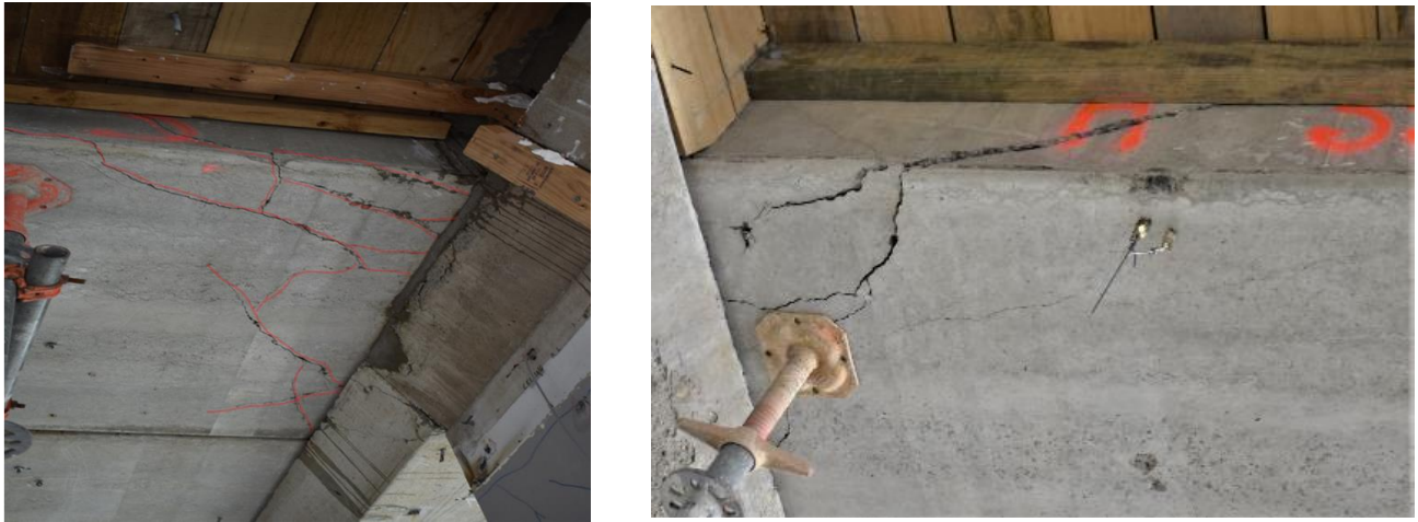
Figure 5. Examples of damage observed in HC floor units with current detailing seated within the plastic hinge region showing cracking of the unreinforced webs of the floor units
