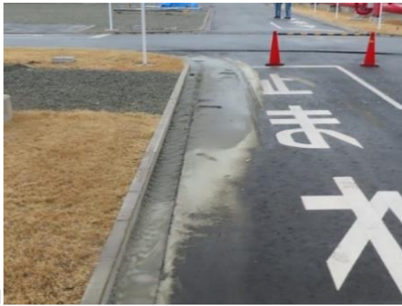
(a) Sand boiling from interface between L-shaped gutters and asphalt pavement
