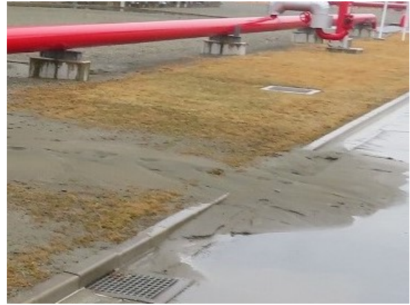
(b) Sand boiling from grass beyond L-shaped gutter
