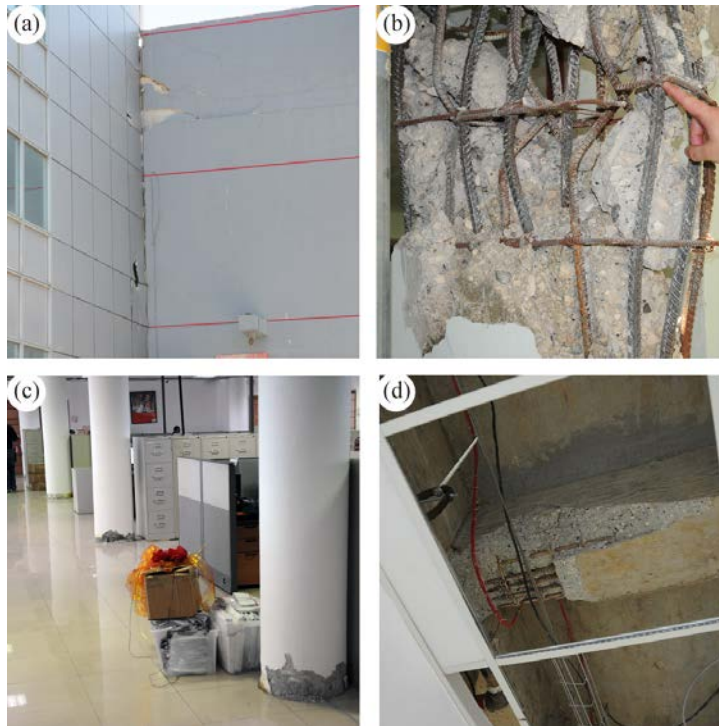
Fig. 14 - a) Evidence of pounding between the high-rise and low-rise parts; b) Damaged parking-structure column; c) 10 th -storey columns on axis 5; d) Damaged beam attached to a wall.
