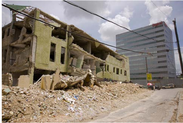
Fig. 11 - The Digicel Building in the background and the damaged “Hopital de Turgeau” in the foreground (both buildings completed just prior to the earthquake).
