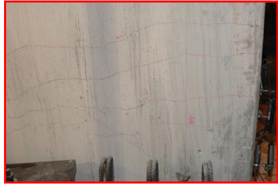
b) Flexural cracks at the base
