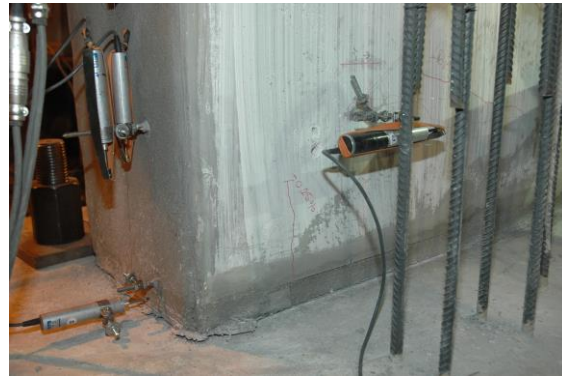
d) Observed base cracks at drift ratio of 0.35%
