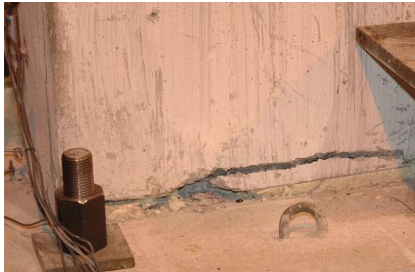
e) Observed base cracks at drift ratio of 0.75%
