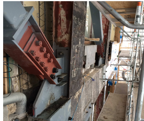
Figure 12 – Installed friction damper
