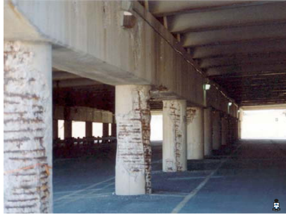
Fig. 1 – Corrosion of spirals in columns
