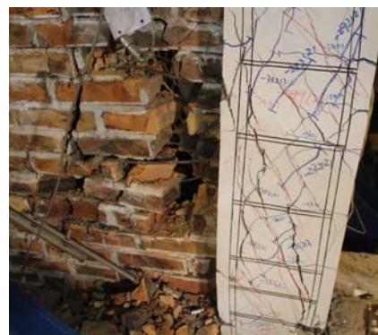
(b) local collapse of masonry infills
