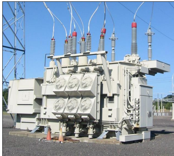
Figure 1, High Voltage Power Transformer
