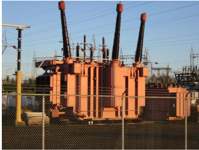
Figure 3, 460 kV Power Transformer
