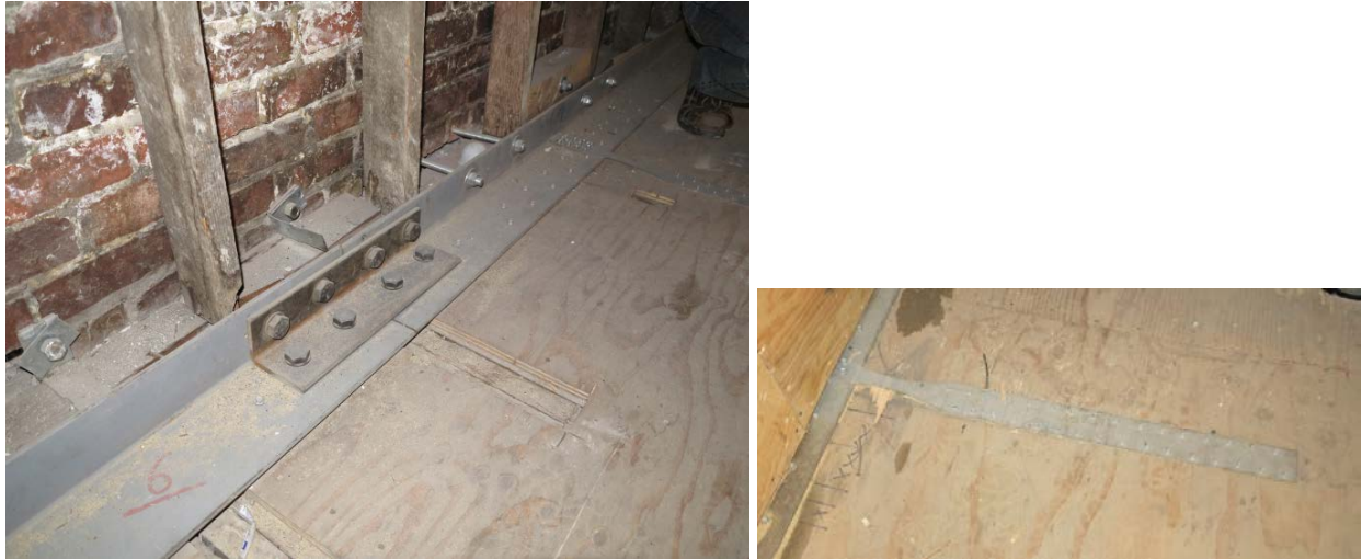
Fig. 3: Diaphragm Upgrading with the addition of Plywood, angles for diaphragm chords and Steel Straps. The steel straps have a potential yielding region to reduce the amount of connection required at the diaphragm side.
