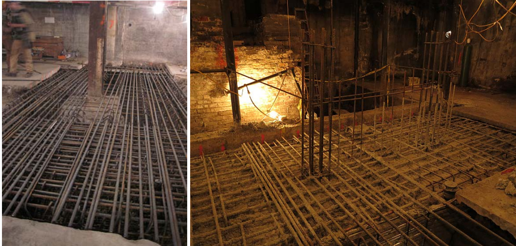
Fig. 4a & 4b: Footing construction in the Marble Arch (Left) and the Hazelwood (Right) .
