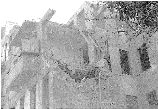
(a) Heavy damage to stone bearing wall buildings in Egypt (EERI, 1992).
