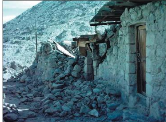
(b) Heavy damage to stone house in Chile (EERI, 2005).
