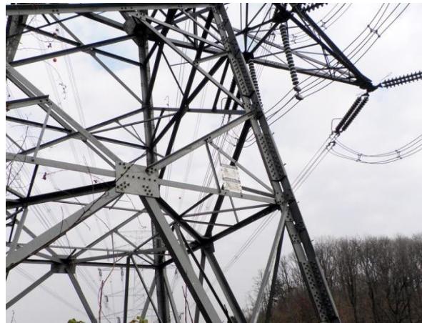
(b) Angle-type transmission tower
