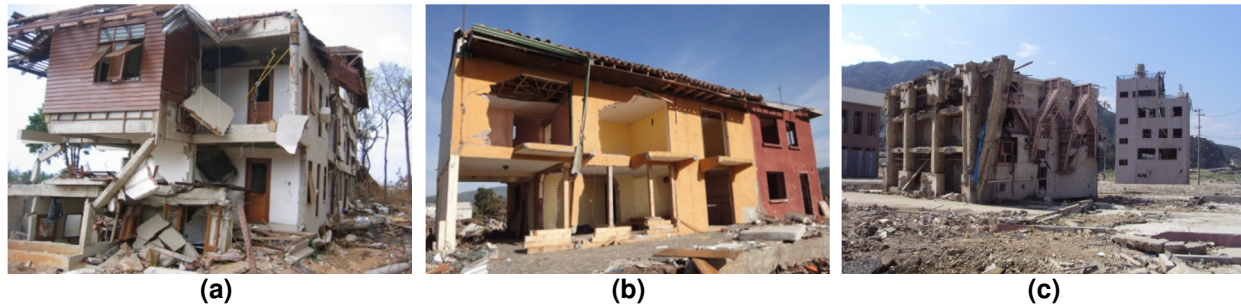
Fig. 1 – Residential structures damaged during tsunami: (a) two-storey concrete building, Khao Lak, Thailand (Nistor et al., 2006); (b) two-storey structure, Pellhue, Chile 2010 (Palermo et al., 2012); and (c) overturned apartment building, Onagawa, Japan 2011 (Al-Faesly et al., 2012)
