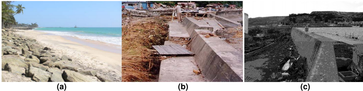
Fig. 5 – Seawall performances during tsunami: (a) seawall in Sri Lanka (Pianc, 2010); (b) Seawall in Taisei, Japan (Pianc, 2010); and c) seawall in Kuji after Tohoku Tsunami 2011 (Chock et al., 2013)
