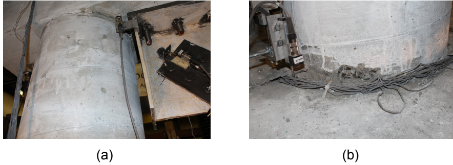
Fig. 9 –Damage in RC Bent Model 2. (a) Horizontal cracks. (b) Spalling of concrete.
