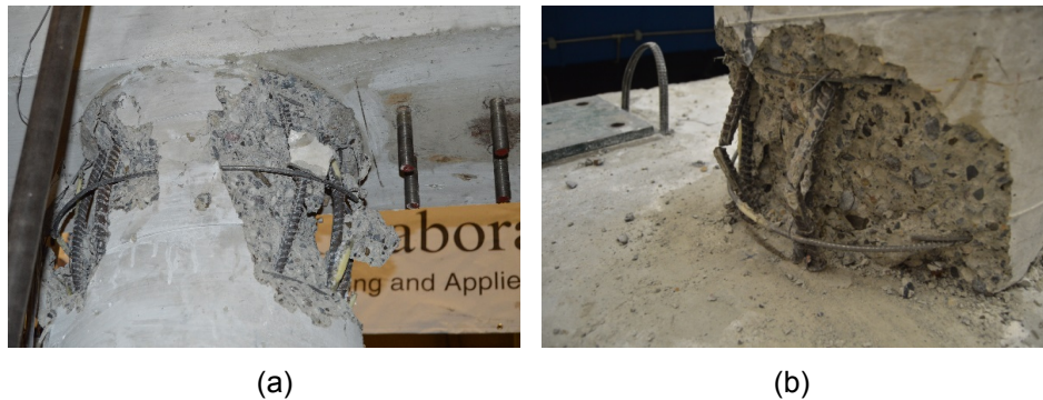
Fig. 12 –Damage in As-built RC Bent. (a) Buckling of steel. (b) Rupture of steel.
