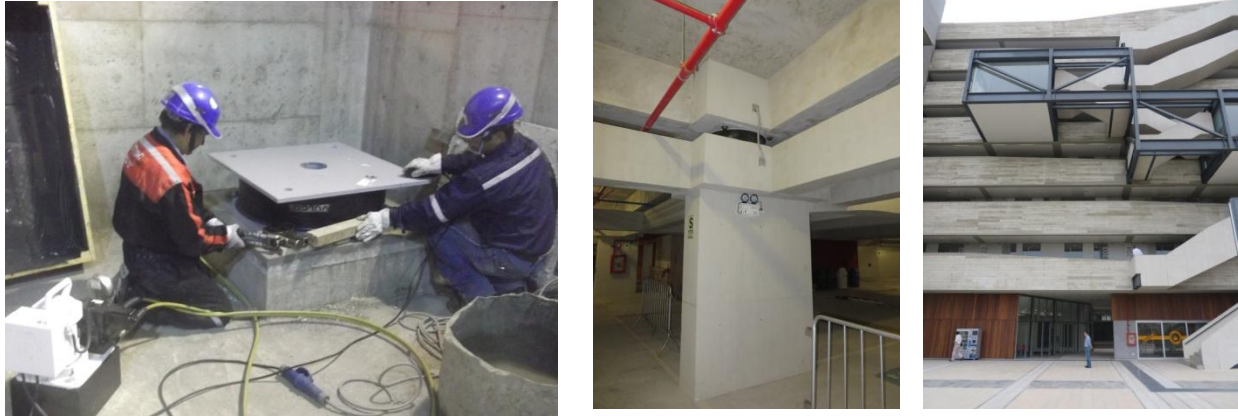
Fig. 6 – Seismic base isolators in university building
