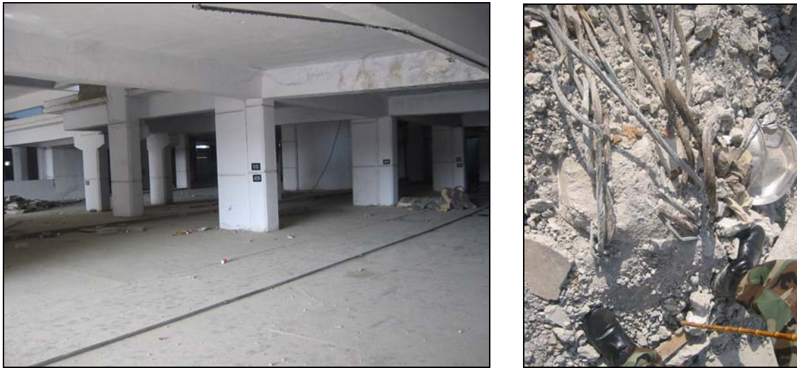
Figure 8. (a) Ground floor of Margala Towers (Islamabad) indicating stronger axis of all the columns aligned in one direction, leaving the system weaker in the lateral direction, (b) Amount of reinforcement and approximate sizes of reinforcing bars at the base of one of the interior columns.
