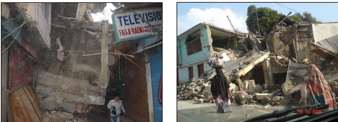
Figure 2. Typical old urban and rural housing units made of brick walls and concrete slabs, Muzaffarabad.
