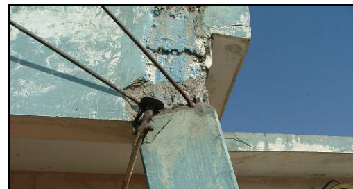
(c) Cold joint and use of unreformed bars
