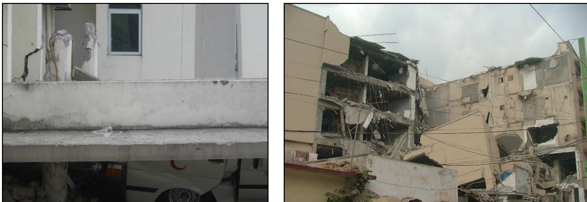
Figure 7. (a) Punching failure of the slab in CMH Hospital. (b) Failure of a hotel building in Muzaffarabad. Poor layout and materials are evident.
