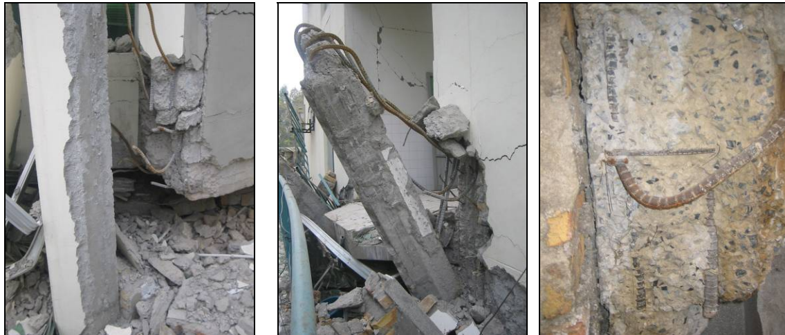
Figure 6. (a) Failure of a beam-column connection, (b) failure of a ground floor columns, and (c) details of the transverse reinforcement, CMH Muzaffarabad. All confirm very poor design and construction practices in the earthquake-affected area even for an engineered critical facility.
