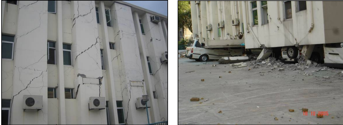
Figure 5. (a,b) Front and back views of the Combined Military Hospital (CMH) in Muzaffarabad. Poor layout leading to soft storey collapse has led to total lack of function and condemnation.
