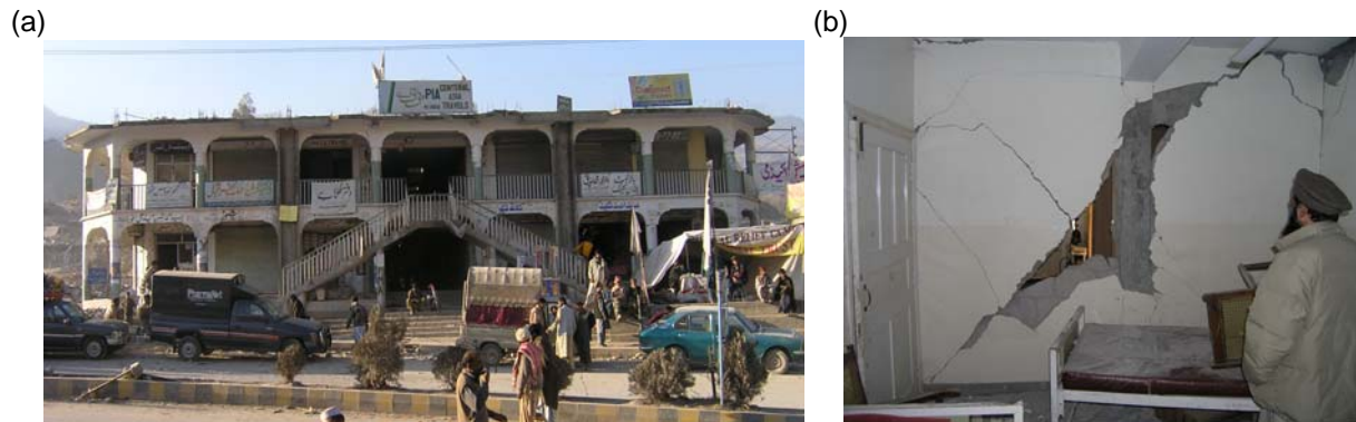
Figure 10. (a) Reinforced concrete hotel building in Balakot; (b) Shear damage to infill walls.
