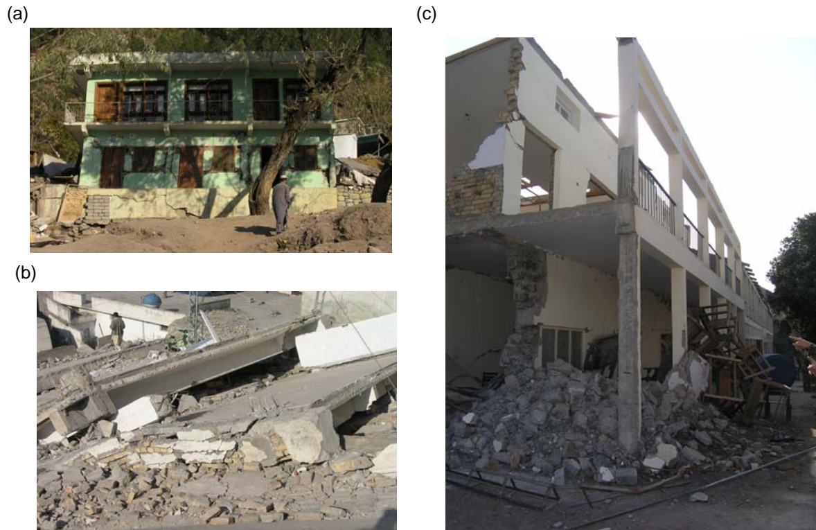
Figure 7. (a) A well-built house in Balakot; (b) A collapsed R.C. building with brick masonry in Muzaffarabad; (c) Partially collapsed R.C school building with brick masonry.
