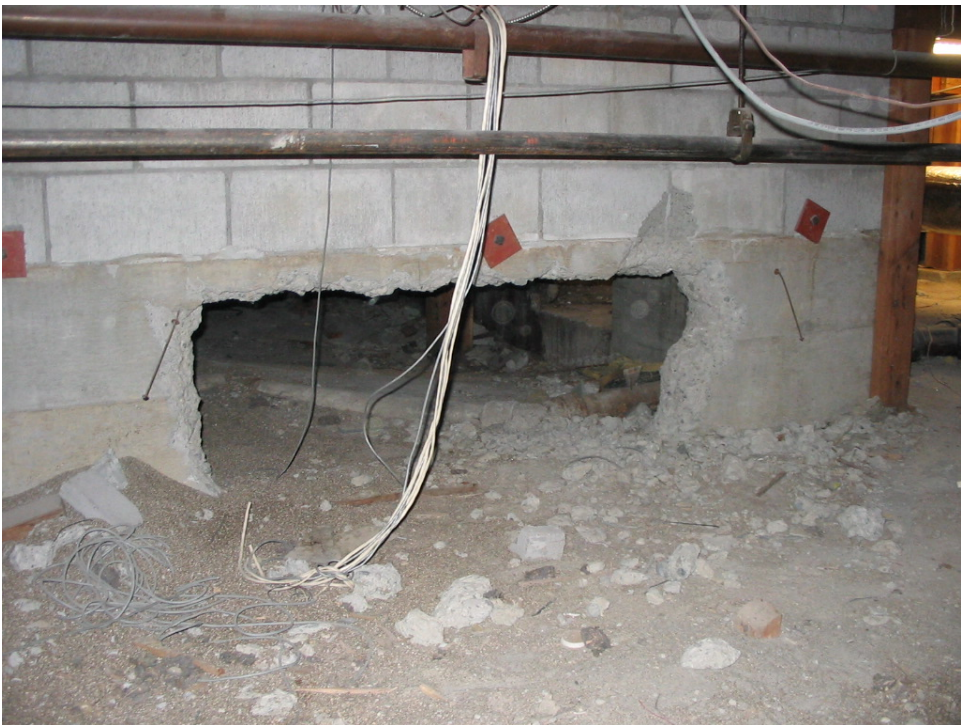
Figure 4 Hole in concrete foundation wall supporting concrete masonry wall in Gym
