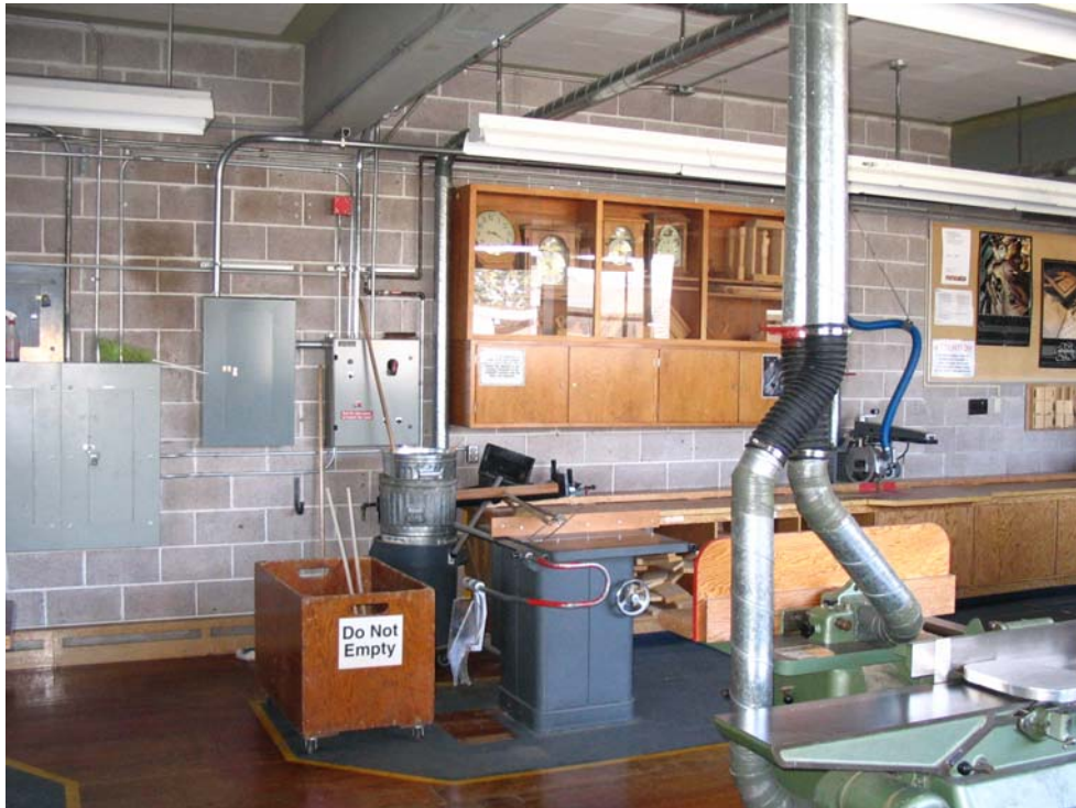
Figure 3 – Wall-Mounted Shop Equipment
