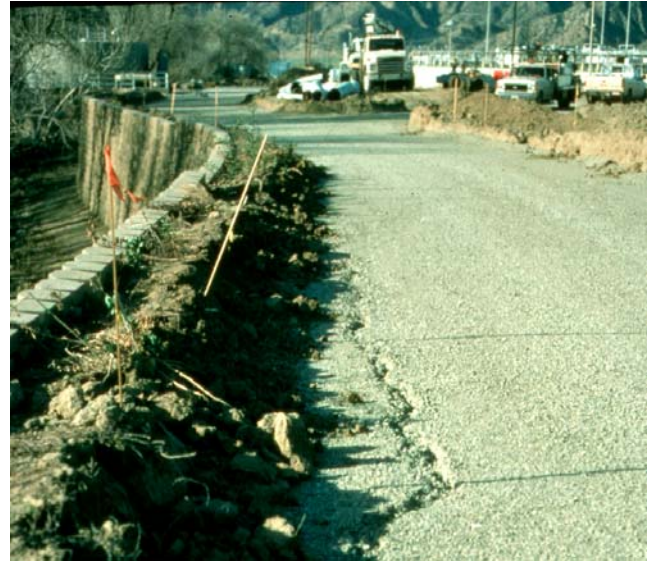
b) photograph taken after earthquake showing cracking at top of wall.
