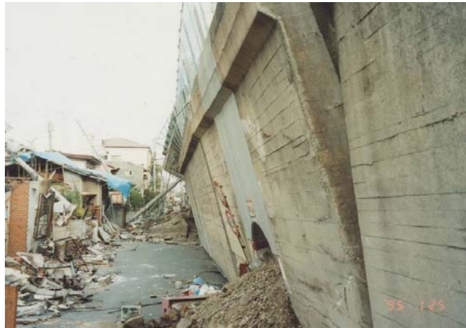
b) example conventional cantilever wall after earthquake
