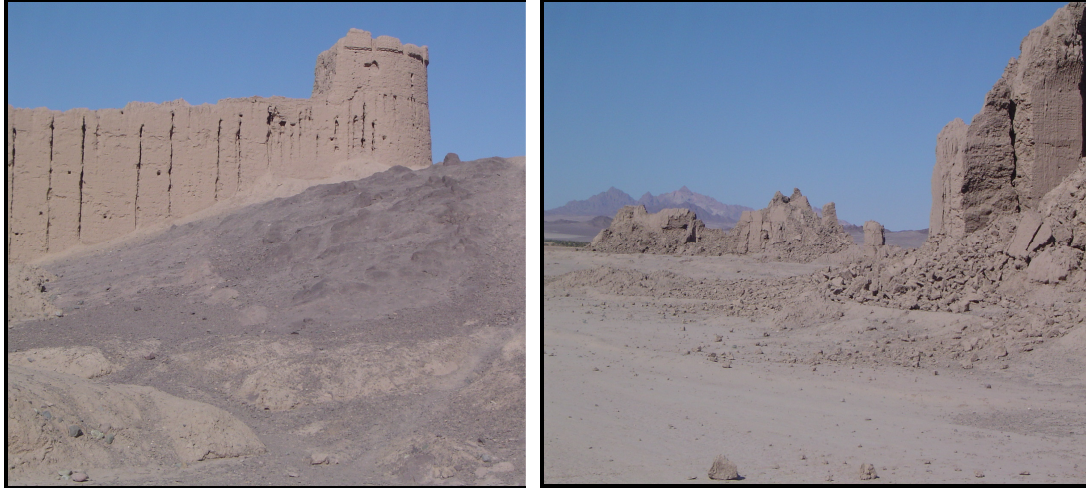
Figure 4. Damage intensity variation of similar buildings on different site conditions in north Bam.
