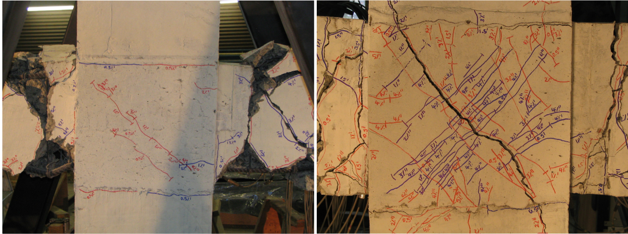
Figure 11. Joint core condition of PVA-1 (left) and PVA-2 (right) at 5% interstorey drift.
