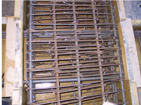
Figure 1. Reinforcement congestion in a beam-column joint core.
