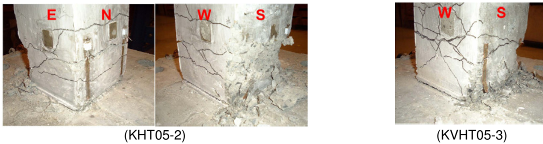
Figure 13. Picture of damage to the base of the columns of KHT05 and KVHT05.
