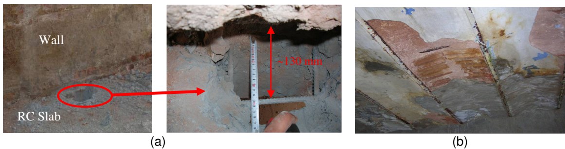
Figure 4. a) The connection of existing walls and reinforced concrete slabs of Block B, b) original vaulted slabs in Block E.
