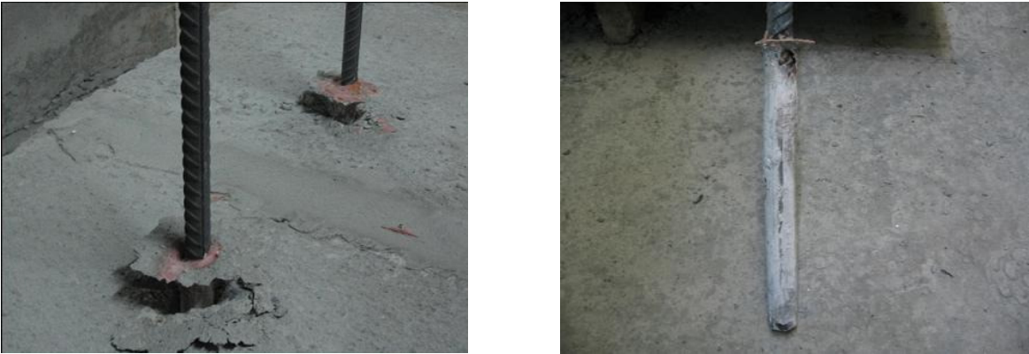
Figure 6. Pull-out failure of anchors bonded with M3 type adhesive.
