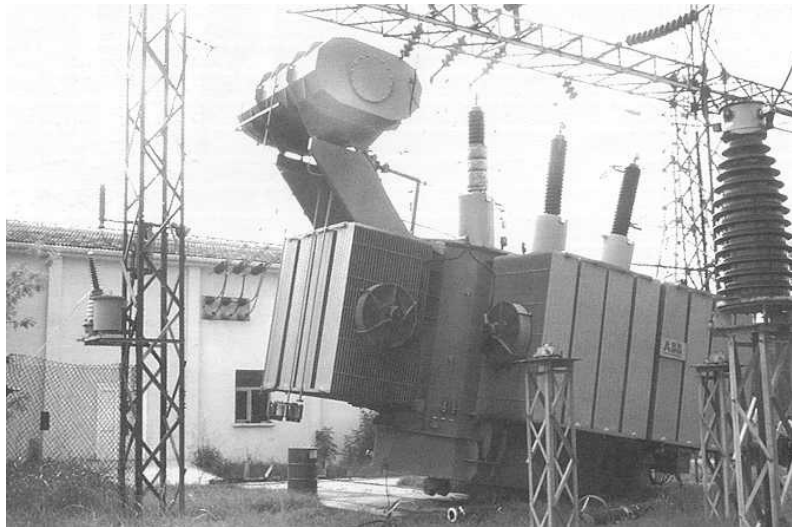
Figure 2. Damage to a transformer caused by support failure (EERI, 1999).
