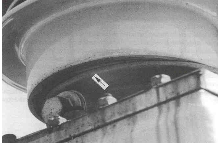
Figure 1. Bushing failure at the flange gasket (ASCE, 1999).
