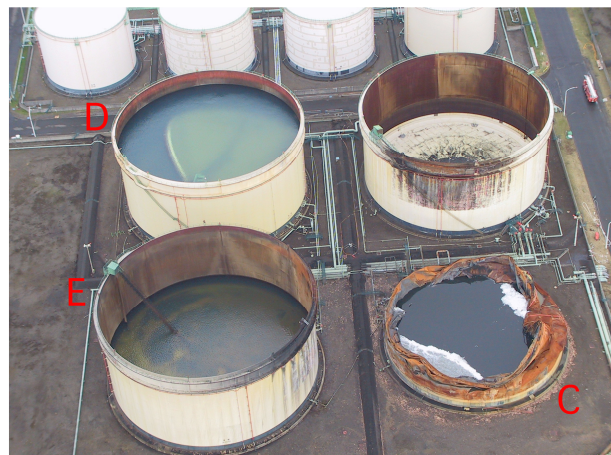
Figure 7. Sunken floating roof (D and E) and pool fire tank (C).
