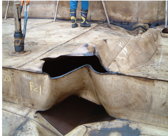
Figure 9. Failure of pontoon.
