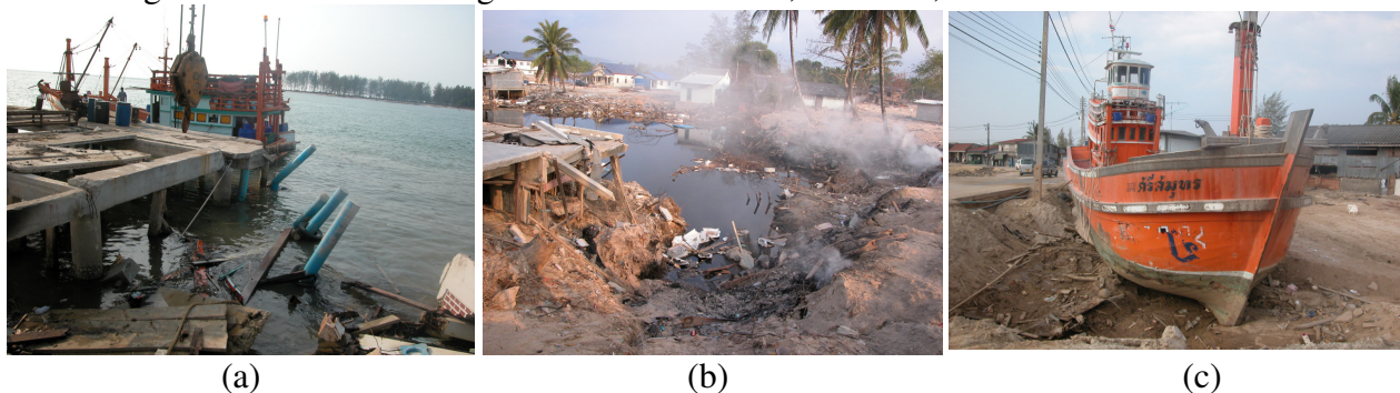
Figure 6. Tsunami-induced damage to the Khao Lak Port, Thailand
