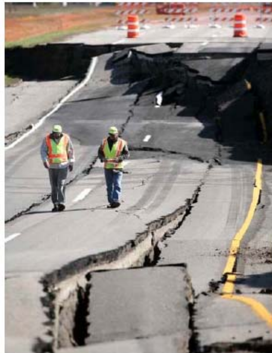
Figure 9. Slope failure on a Minnesota highway that was successfully predicted using Wireless Shape-Acceleration Arrays (Photo courtesy Mn/DOT).
