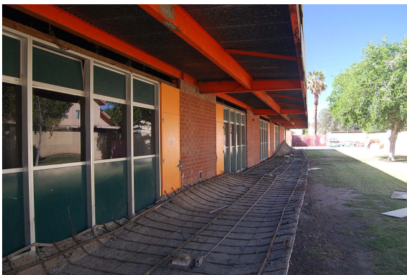
Figure 1 Jefferson Elementary Stucco Soffit Collapse in the Baja Earthquake
