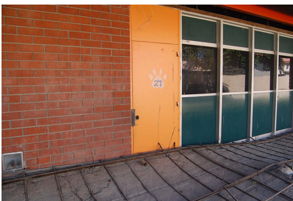
Figure 2 Soffit collapse blocked the classroom doors and sheared off some doorknobs.
