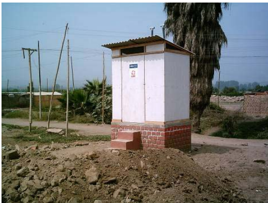
a) Dry hole latrine
