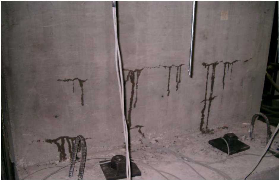
Figure 5: Leakage at the back face of the wall after yielding of the front side vertical reinforcement.
