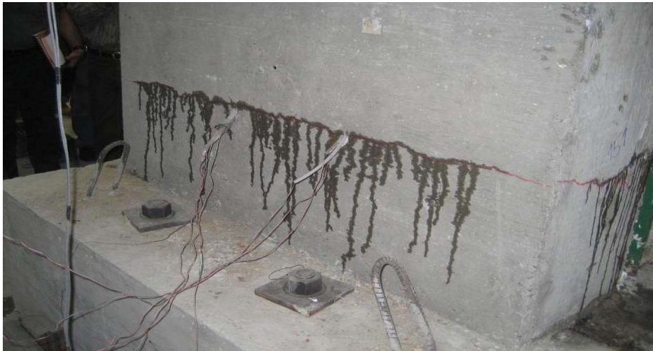
Figure 8: Leakage at the back side of the wall at the initial stage of the leakage test.
