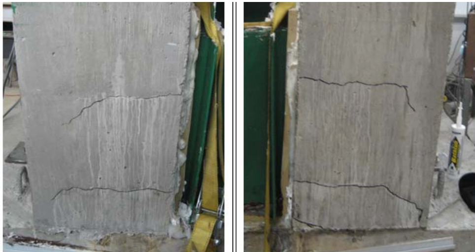
Figure 4: Cracking of the side faces of the wall after the test.
