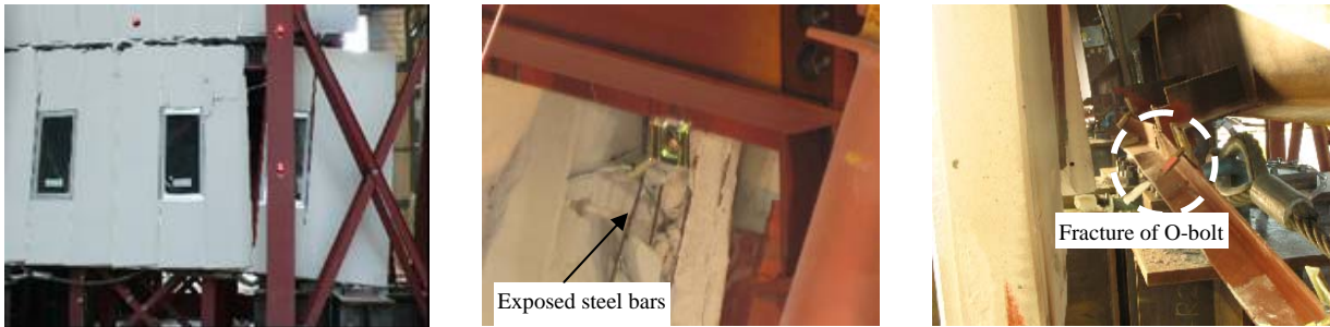
(a) Damage to the ALC panels (b) Damage B (c) Damage C Figure 3. ALC panels after test by 1.0 Takatori records
