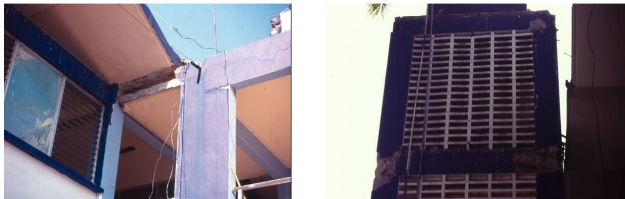
Figure 2. Observed damage in the Health Ministry Hospital at Manzanillo during the October 9, 1995 Manzanillo Earthquake
