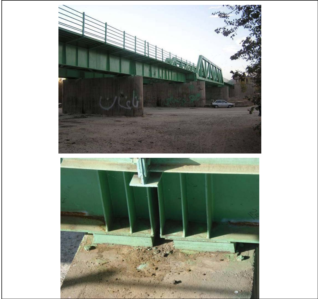
Figure 3. Gap over the pier
