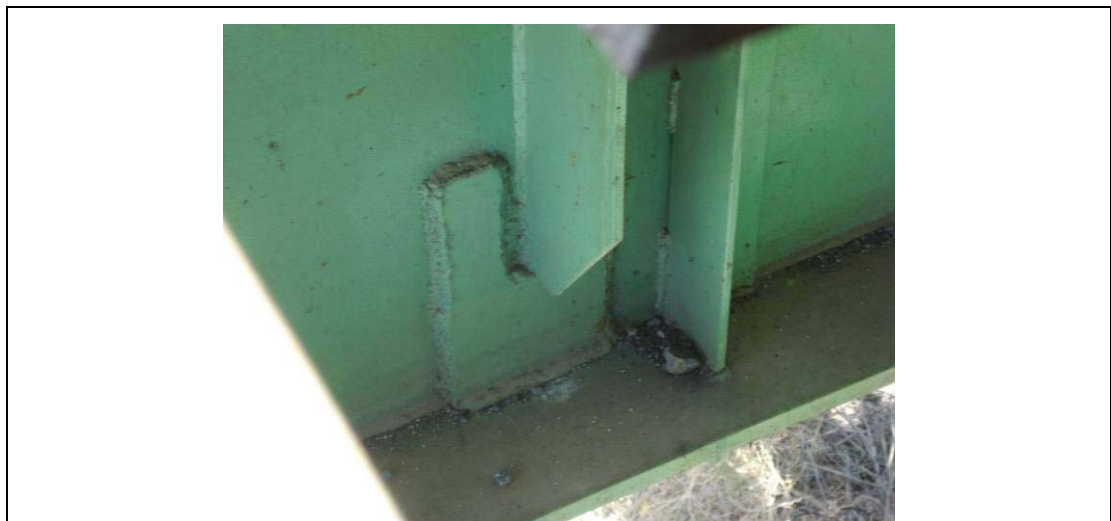
Figure 6. Stiffeners in the transverse girders (other plates have been added later)
