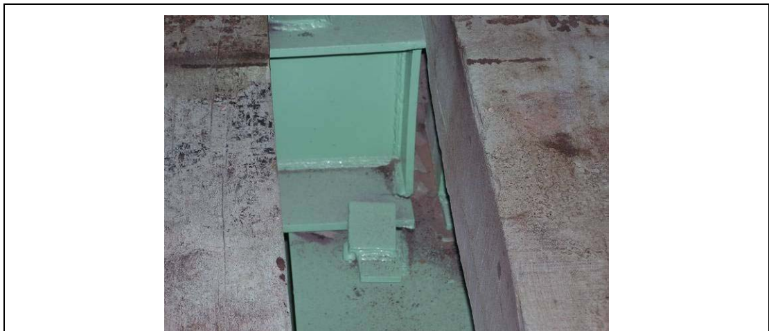
Figure 4. Crack in the connection between longitudinal beam and transverse girder
