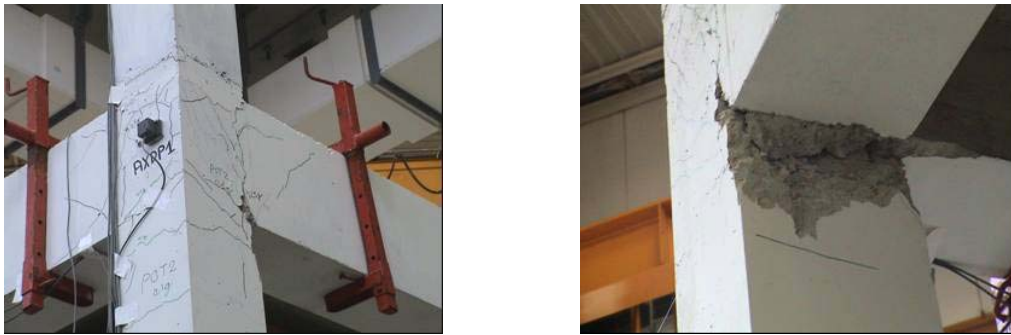
Figure 2. Damage in joints and columns after the test PGA=0.4g (notice bond-slip failure at the column-beam interface)
