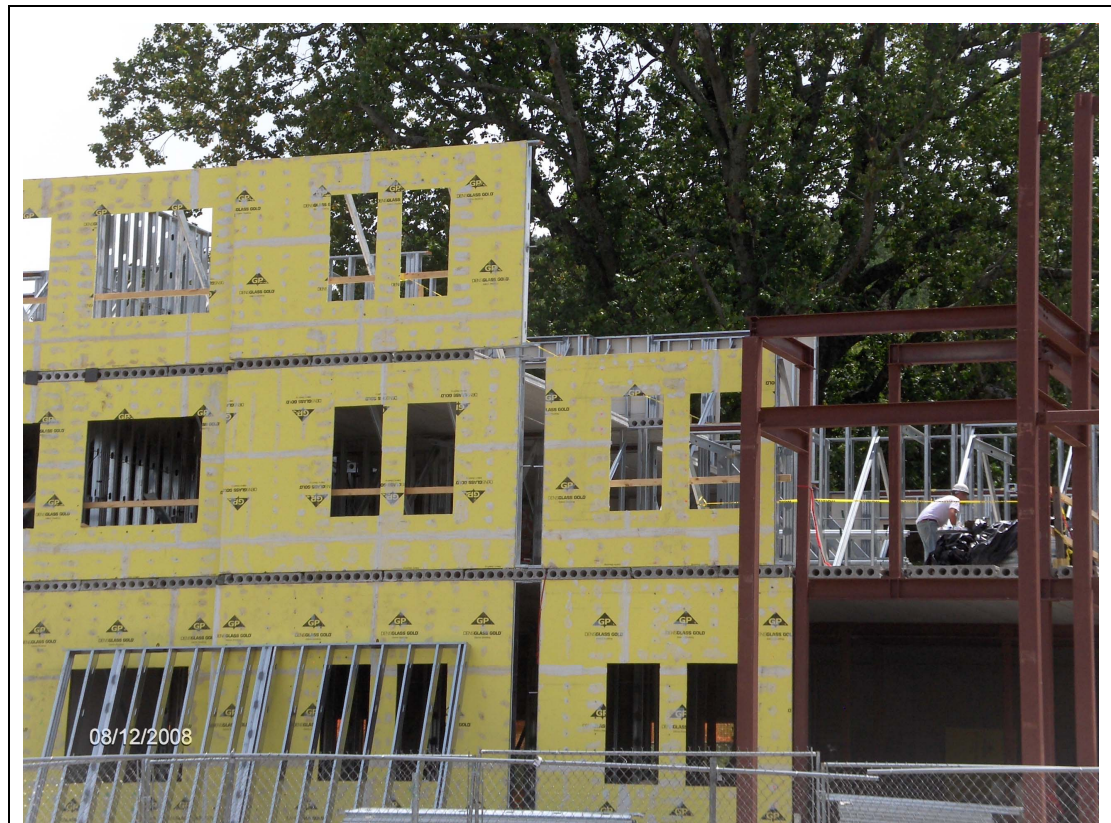
Figure 1. A building under construction with steel stud walls and concrete plank floors that does not correspond to one of the standard building types.
