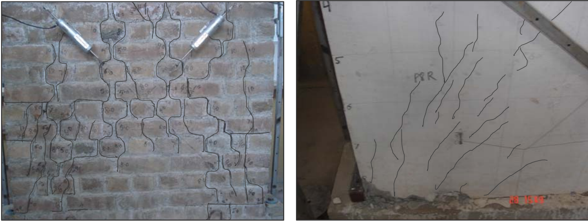
Figure 7. Final damage photograph of specimens P8 (left) and P8R (right)
