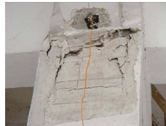
Figure 7. Crushing of column ②-⑧ at the load step 15
