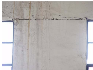
Figure 9. Horizontal crack in wall ① at the load step 23
