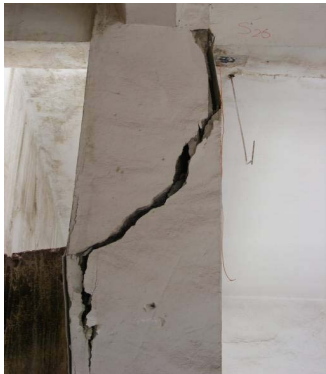
Figure 6. Shear failure of column ③-⑧ at the load step 23
