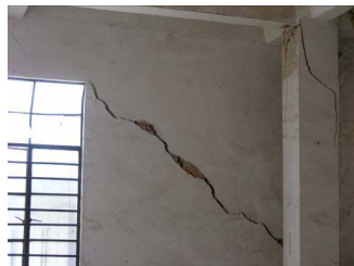
Figure 8. Inclined crack in wall ① at the load step 23
