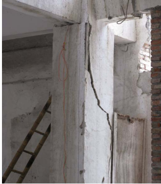
Figure 4. Shear failure of column ③-⑧ at the load step 15
