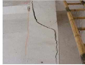
Figure 5. Shear failure of column ②-⑧ at the load step 23
