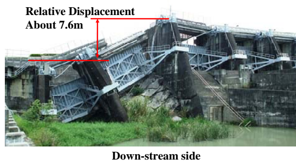
Figure 1. Existing Dam damaged by Surface Fault Displacement
