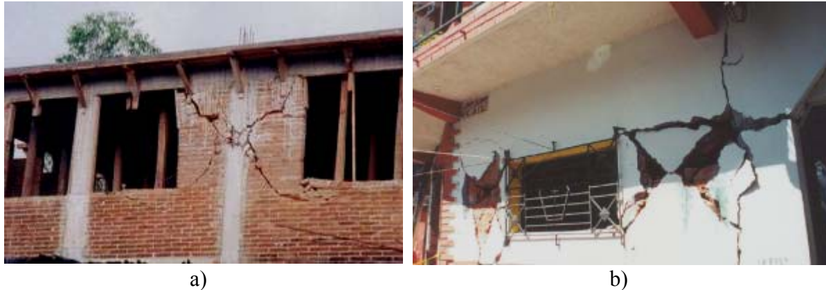
Figure 4. In-plane shear damage of confined masonry construction: a) the 1999 Tehuacan, Mexico earthquake (Alcocer et al. 2001), and b) the 2001 El Salvador earthquakes (EERI 2001).
