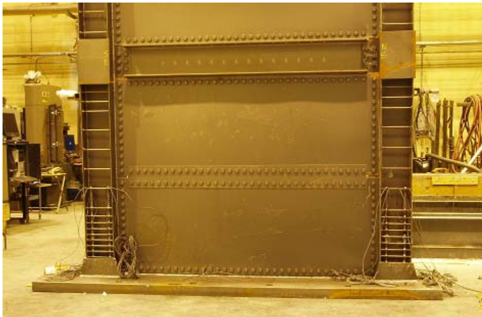
Figure 5. First floor of steel plate shear wall with PEC columns before casting concrete
