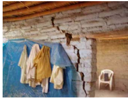
Figure 12 Heavy cracks in the adobe house of Figure 10
