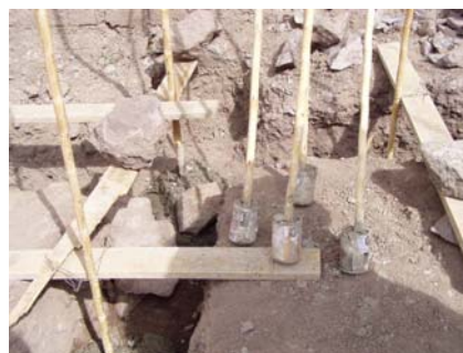
Figure 14 Modified method of anchorage in Huangascar. Vertical canes are fixed to empty cans in advance
