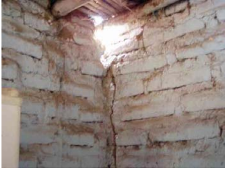
Figure 11 Broken walls of the adobe house of Figure 10
