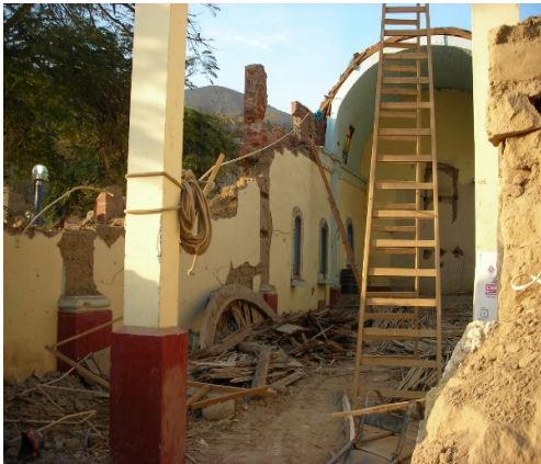
Figure 7 Heavily damaged church in Zuniga Wall: adobe, Vault roof: Quincha
