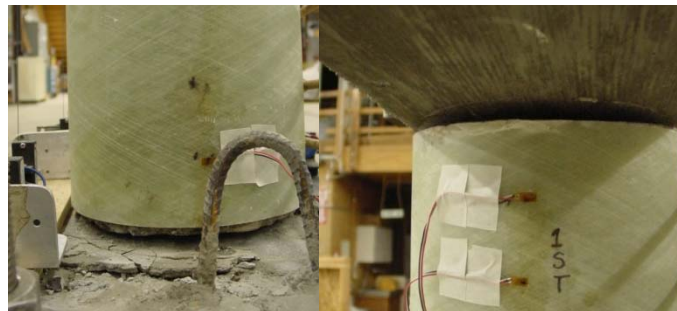
Figure 8: Opening of the top and bottom interface joints for the north column of Specimen F-FRP1
