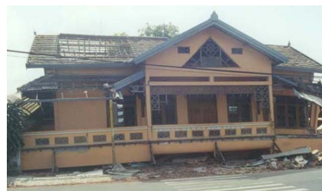
b. Shop houses suffered severe damage after Yogyakarta earthquake 2006
