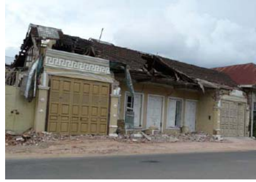
b. After Padang Earthquake 2009
