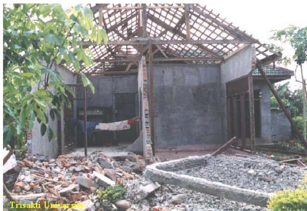
a. After Bengkulu earthquake 2000
