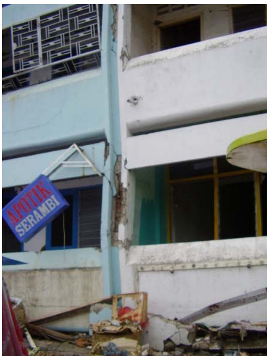
a. Shop houses suffered severe damage after Aceh earthquake 2004
