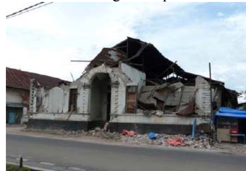
d. After Padang Earthquake 2009
