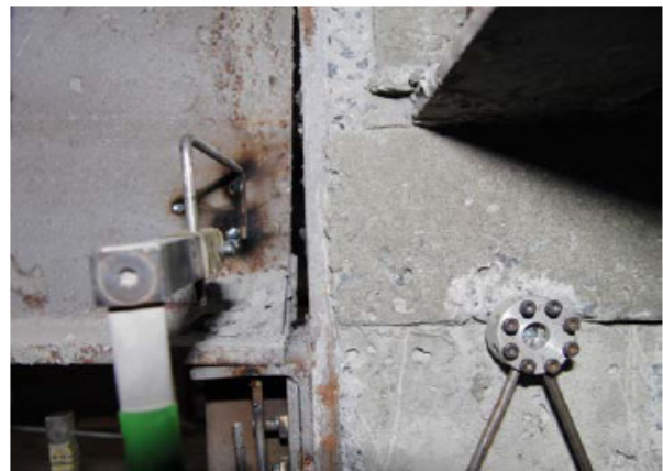
Fig 16. Fracture of bolts between beam and angle
