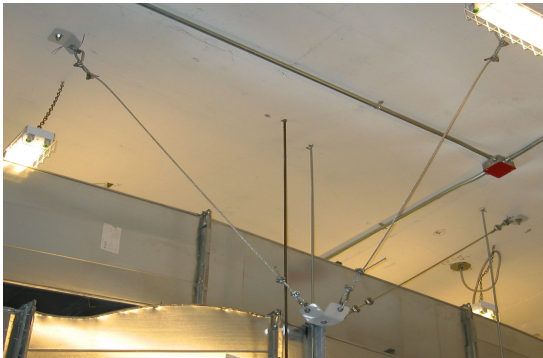
Figure 5a. Cable restraints on duct.
