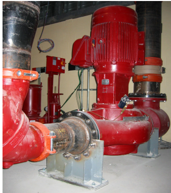
Fig.4 – Inline pump supported with stands
