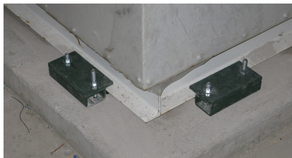
Figure 3. Rigid restraint equipment snubbers.
