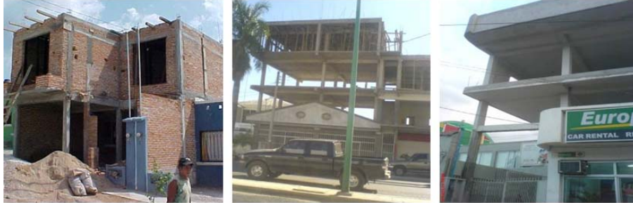
Figure 2. Examples of structures with soft floor and problems of abrupt change stiffness and mass in the city of Tuxtla Gutierrez, Chiapas.
